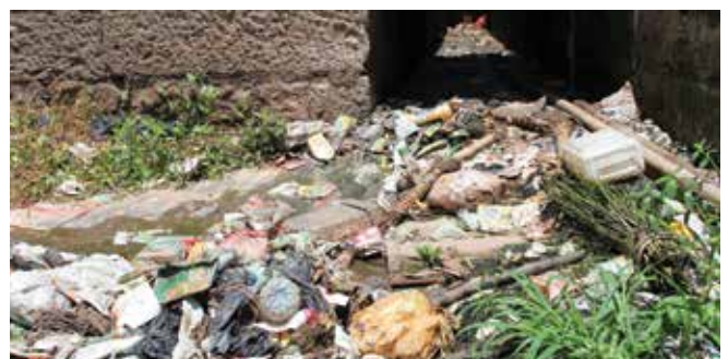
An uncovered school septic tank in Zhong County, Chongqing Municipality
